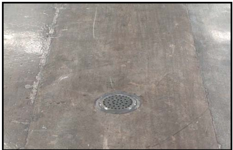
Heat is redirected to floor heat vents at pool facility
